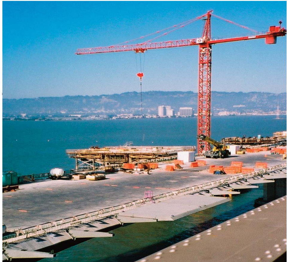
Initial deck installation of the Alexander Zuckermann Bay Bridge Path in July 2005.
