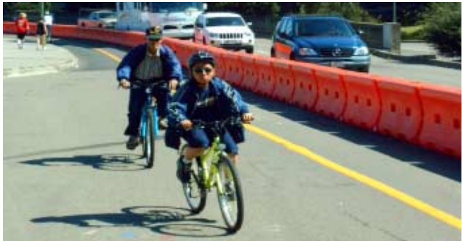
New pavement installed for bicyclists on 12th St dam at the foot of Lake Merritt. Water-filled barriers complete the Interim 2-Way Path until construction begins to replace the 12 lanes of the "World's Shortest Freeway" with a 6-lane Lake Merritt Boulevard, adding acreage to the park and bike lanes to the road.
