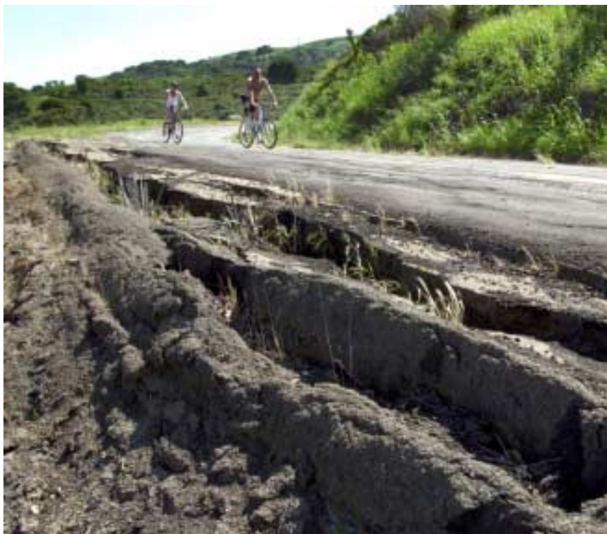
Large sections of roadway slough off during winter rains — see article page 3.
