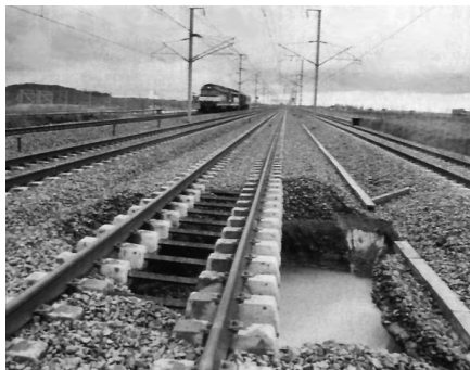
At 182 mph, this was the scene of the world's fastest and most spectacular derailment. It occurred on this TGV line in 1992 when, after a period of heavy rains, a sinkhole opened up under the tracks, possibly caused by a trench from World War I. The TGV's articulated design kept the train from jackknifing or leaving the track bed. (Photo: Jean-Marie Hervio / Le Parisien Libéré; see http://mercurio.iet.unipi.it/tgv/wrecks.html for more on the TGV accident history.)
